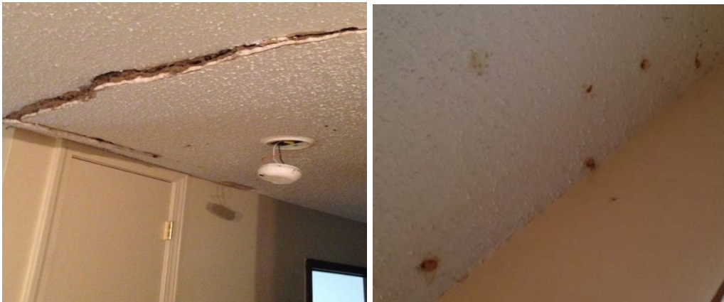
Illustration 3: Unit 1 with cracked ceiling and insect nests
