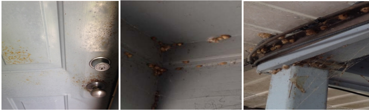
Illustration 2: Unit buildings with rust on entry doors and insect nests under porch areas
