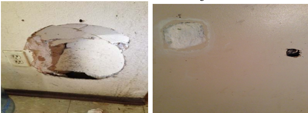
Illustration 4: Unit 1 with wall damages
