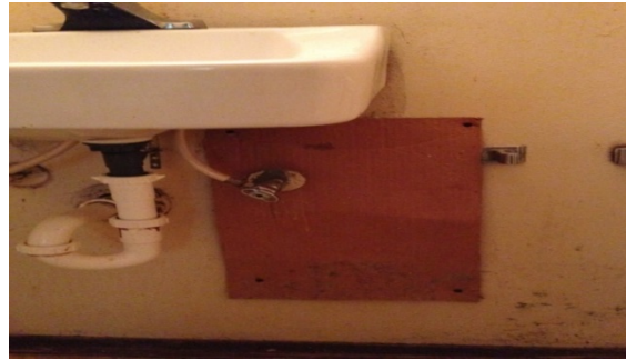
Illustration 5: Unit 2 with incomplete plumbing work
