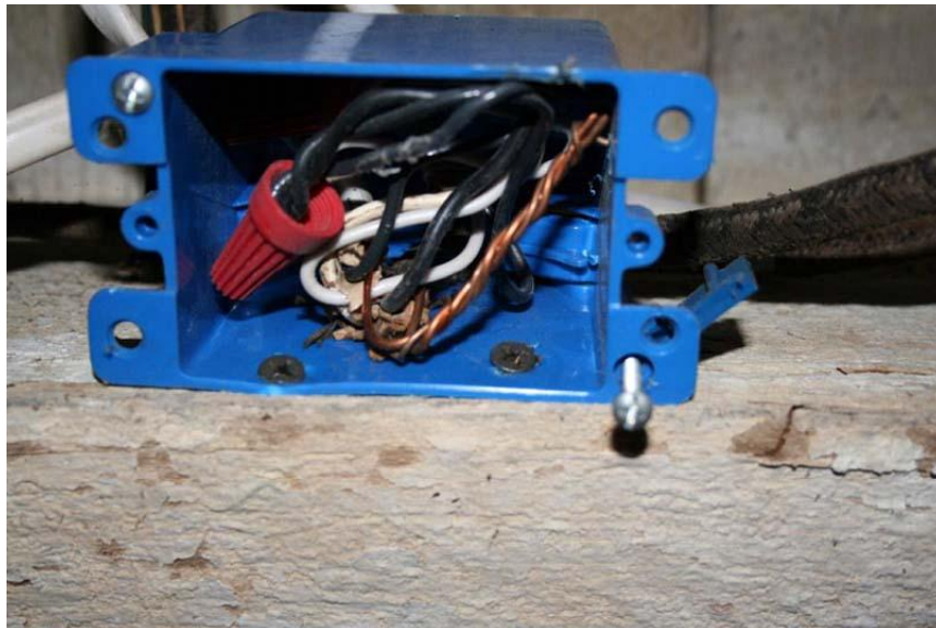
Inspection V21104: Cover is missing on junction box. This violation was not identified during the Authority's December 18, 2008, inspection.
