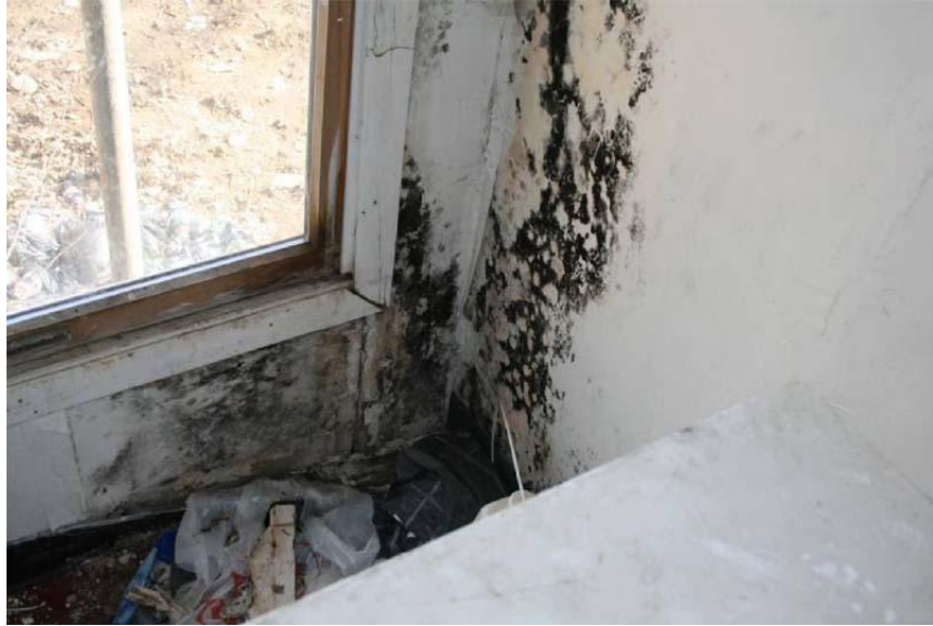
Inspection V51089: Mold is present from a water leak. This violation was not identified during the Authority's August 25, 2008, inspection.
