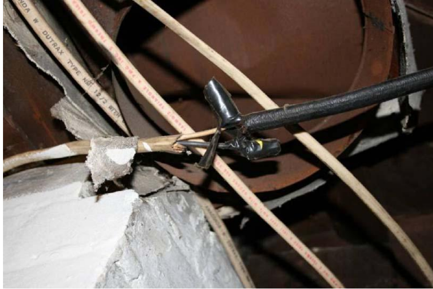
Inspection V20045: Electrical connection is made outside of the junction box. This violation was not identified during the Authority's September 5, 2008, inspection.
