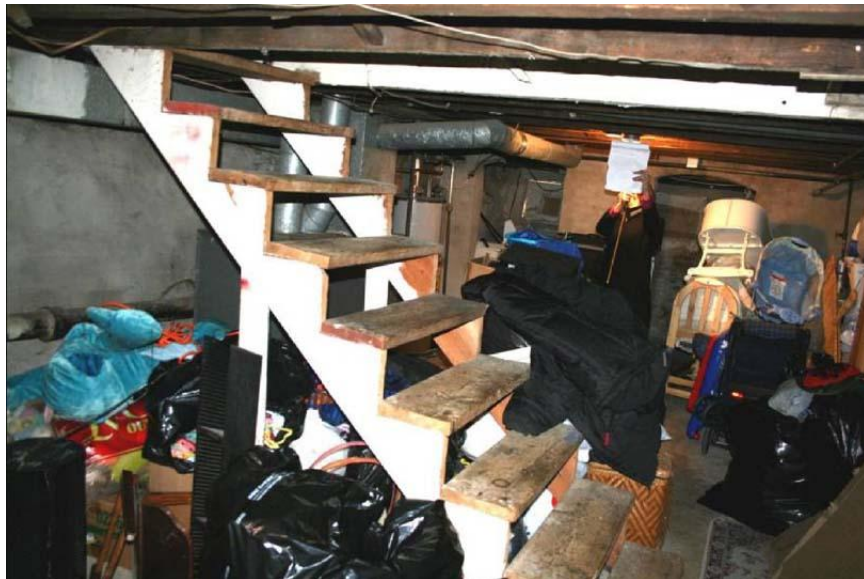
Inspection V20039: Basement stairs need a handrail. This violation was not identified during the Authority's January 26, 2009, inspection.
