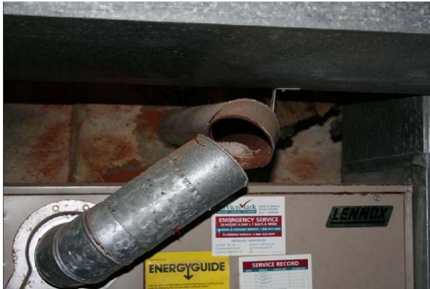
Inspection V38083: Flue pipe is rusted/disconnected from the furnace and is releasing fumes into the basement. This violation was not identified during the Authority's January 6, 2009, inspection.
