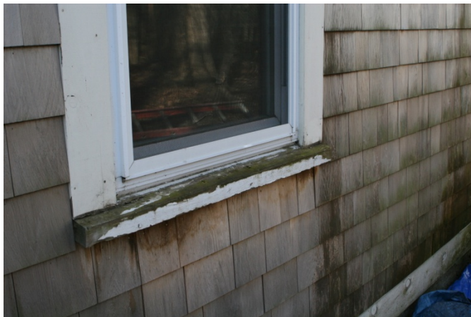
Mildew and rotten window sill
