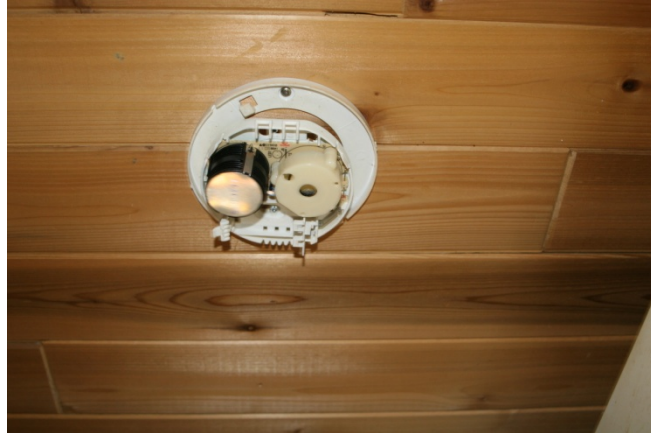
Damaged smoke detector
