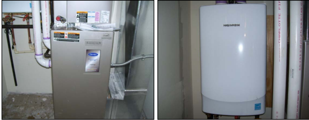
New high-efficiency furnaces (left) and tankless water heaters (right) were installed in units at the Southbridge family development (ongoing).
