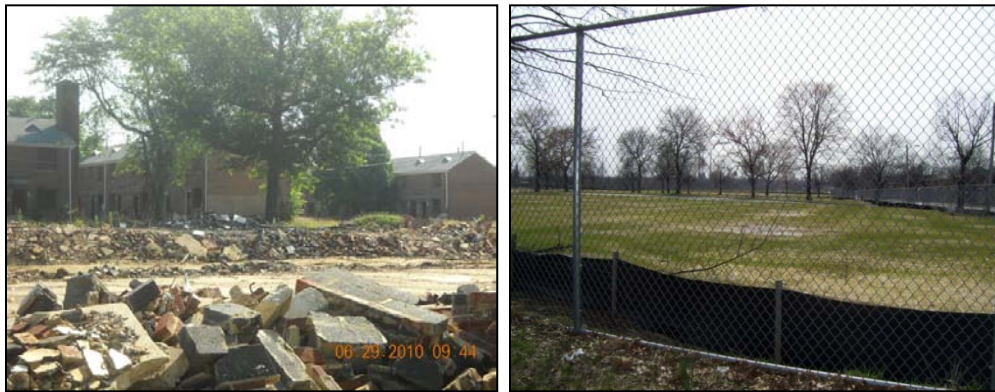
Before (left) and after (right) pictures illustrate the demolition of public housing units at Riverside (completed).
